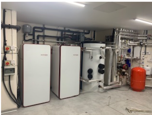
Examples of Heat Pumps and Heat Storage Vessels
