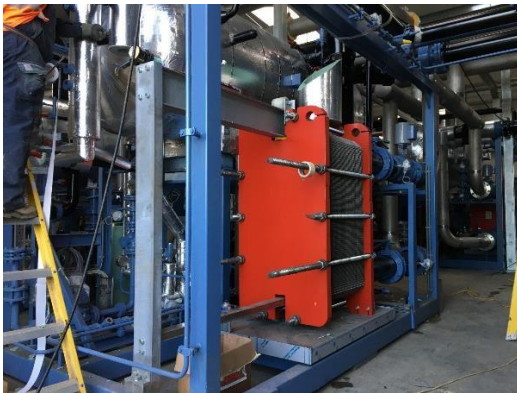
Borehole water plate heat exchanger
