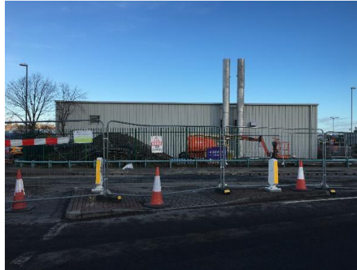
New Heat Pump Energy Centre
