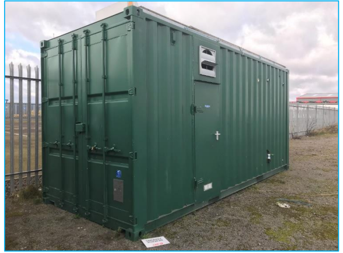
Containerized anaerobic digestion unit
