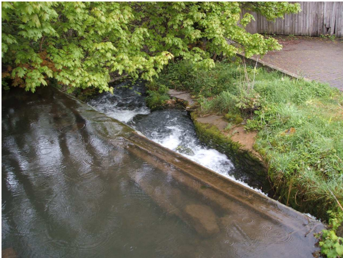
Figure 7 : Upturned channel on part of the weir crest
